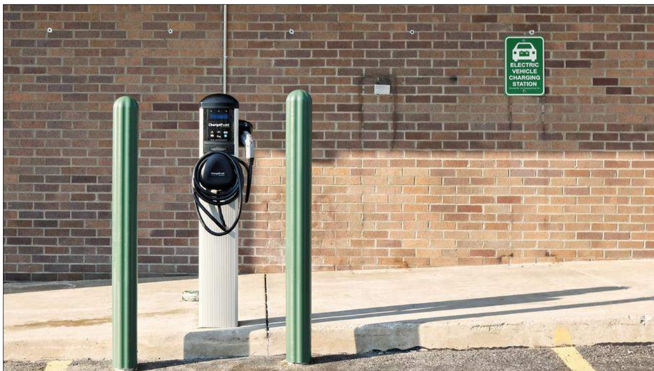
Figure 18: Level 2 Charger at Walgreens, Akron, OH
