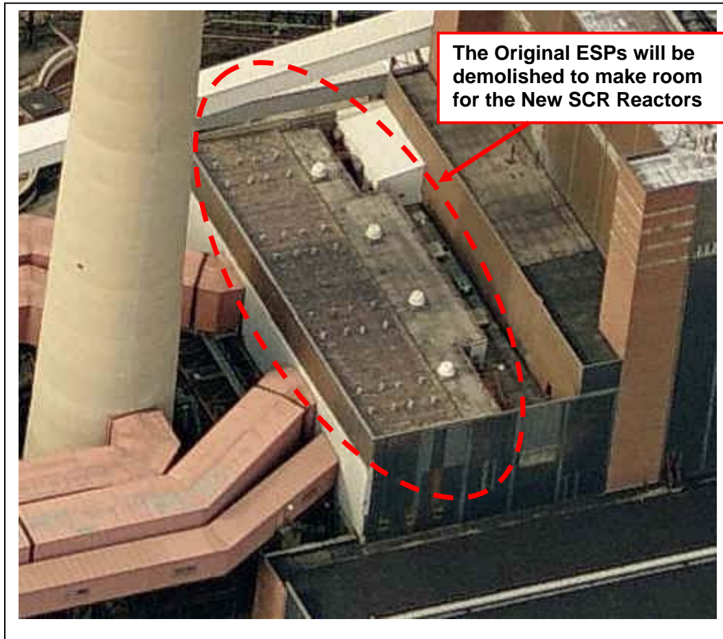
Figure 5.1-2: View of Avon Lake Unit 9 Showing Original ESPs
