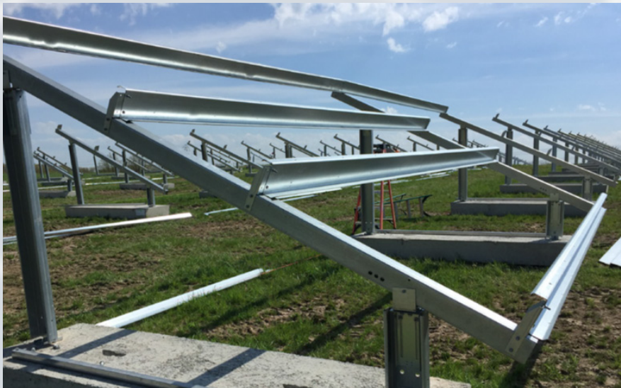
Figure 2. Racks For Solar Panels, Brooklyn, Ohio Site (Ref. 3)
