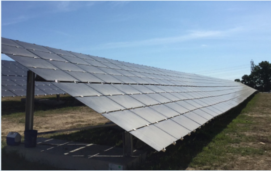
Figure 3. Installed Solar Panels, Brooklyn, Ohio Site (Ref. 3)
