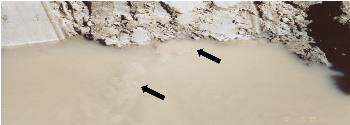
Figure 7-4 Example seepage through the foundation
