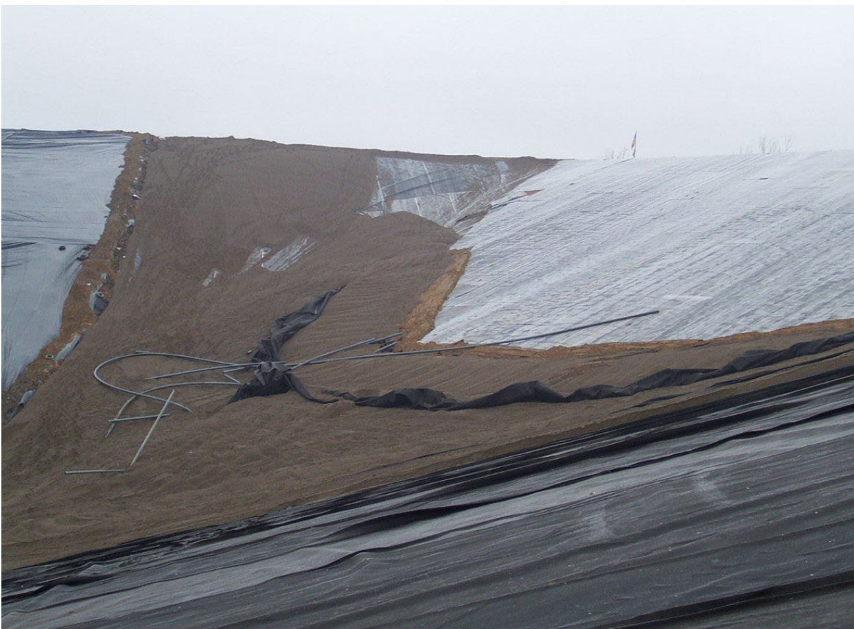
Figure 1-2, Failed slope at an Ohio landfill between textured geomembrane and GCL covered with 1 ft. of pea gravel on 3 to 1 slope after being placed with a Caterpillar D8 (14.7 psi) pushing up slope. Some movement was seen during gravel placement but by the next day the slope had completely failed.
