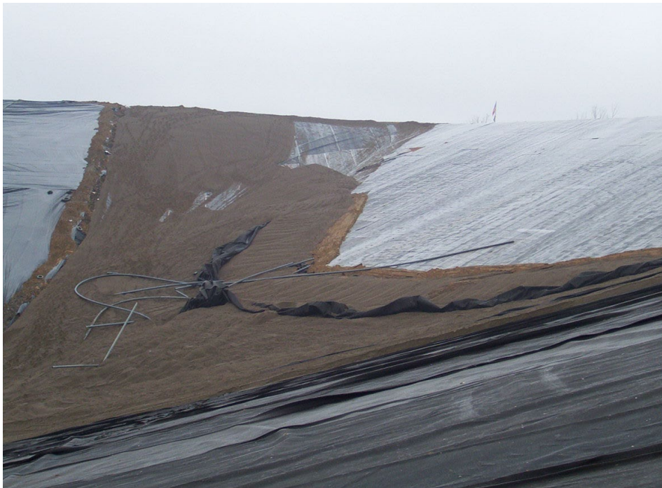
Figure 9-7, Failed slope at an Ohio Landfill between textured geomembrane and GCL covered with 1 ft. of pea gravel on 3 to 1 slope after being placed with a Caterpillar D8 (14.7 psi). The calculated factor of safety for equipment loading conditions was 0.827 ( \approx a=20 psf, \delta=23^\circ ) and the calculated factor of safety for static conditions after the equipment was removed using large displacement shear strengths was 1.23 ( \approx a=27.9 psf, \delta=16.9^\circ ).
