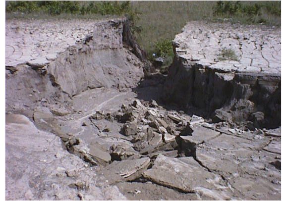
Figure 8-10, Looking through the failed containment berm of a storm water retention basin located in Cuyahoga County. The outlet was plugged, causing the phreatic surface in the basin to become unexpectedly high. As a result, it overwhelmed the shear strength of the soil materials used to construct the berm and caused it to collapse.
