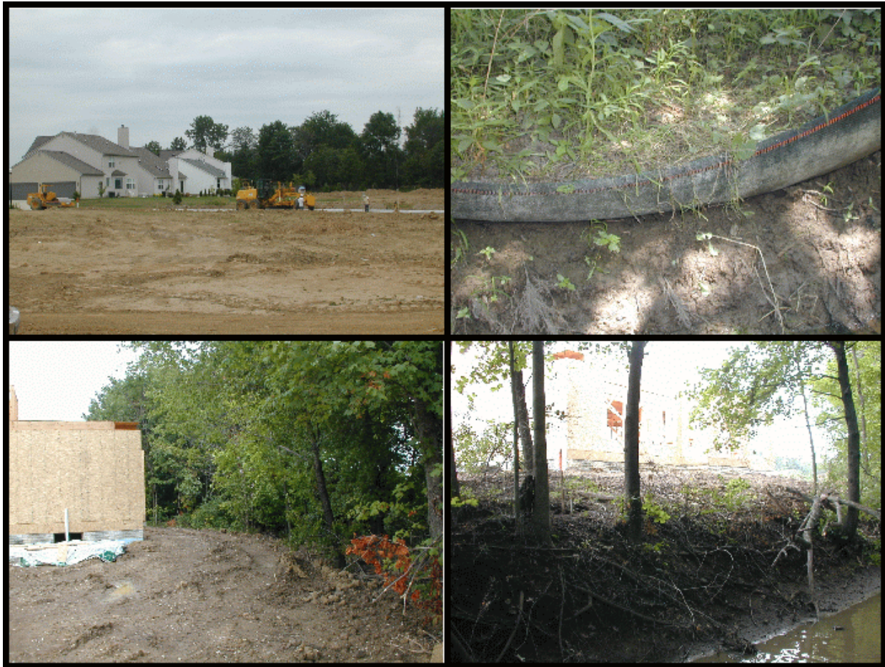
Figure 43. Construction in the Rocky Fork basin. Upper left, cluster development in the vicinity of Walnut Street. Upper right, a properly constructed silt fence along the bank of Sugar Run. Lower panels, new home construction lacking proper erosion controls, and encroaching on and destroying the riparian zone.
