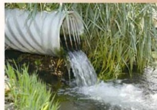
Figure 1: Subsurface tile drain outlet (courtesy of the Leopold Center for Sustainable Agriculture, Jerry DeWitt)
