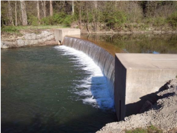
Figure 32: A dam on the East Branch at RM 2.0 (Kirtland Country Club) may impede fish migration across the structure and contribute to nonattainment of the East Branch upstream (RM 2.4). (CRWP, 2011)
