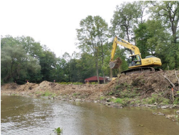
Figure 18: Before restoration at Holden Arboretum: 10-foot-tall levee blocked floodplain access
