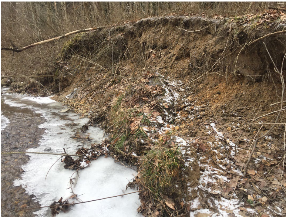
Figure 37: Streambank erosion and siltation on Sunnybrook, a tributary to the East Branch.
