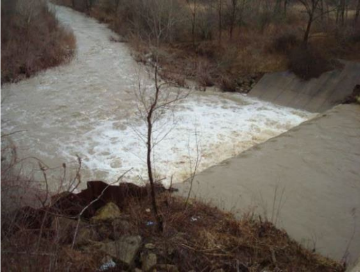
Figure 35: Sheet pile dam and concrete dam is a fish barrier on the East Branch at RM 15.1
