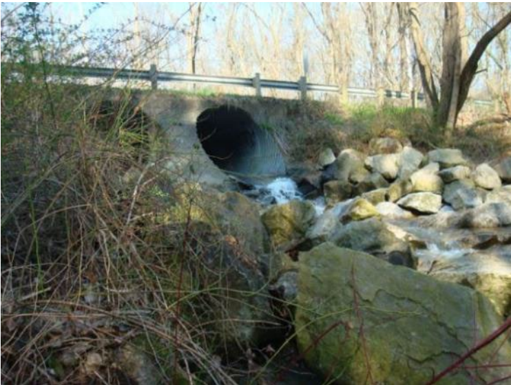
Figure 36: Unnamed tributary to East Branch at RM 15.35 is impaired by a perched culvert that acts as a fish barrier.
