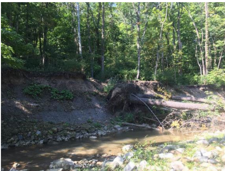
Figure 28: Streambank erosion at approximately East Branch RM 14.7. (CRWP, April 2012)
