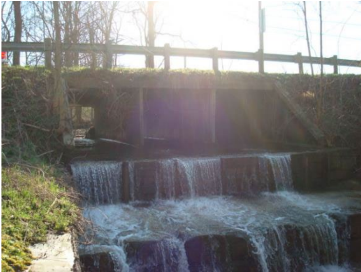
Figure 33: The Heath Road bridge over Harris Creek is a fish migration barrier to upper reaches of this tributary.
