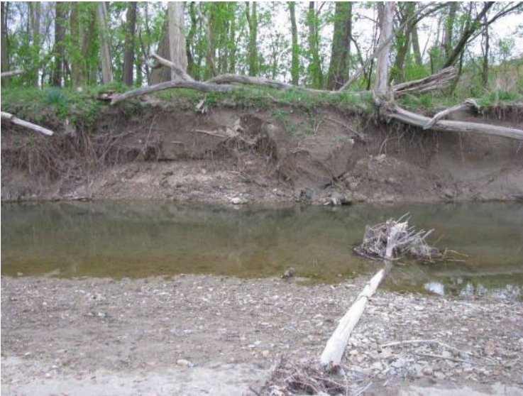
Figure 24: Streambank erosion along the East Branch near its mouth (facing left bank downstream). (City of Willoughby, May 2012)
