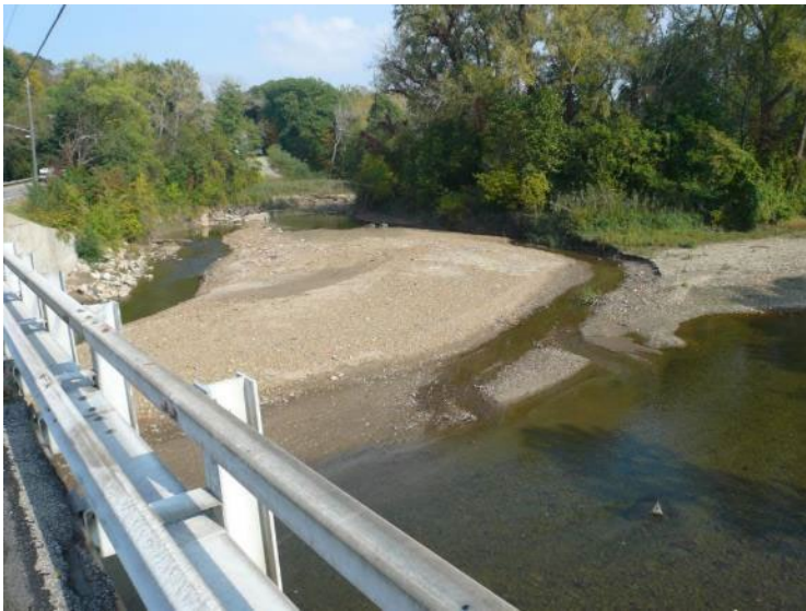
Figure 23: Streambank erosion and material deposition at the confluence of the East Branch with the mainstem of the Chagrin River. (CRWP, July 2013)
