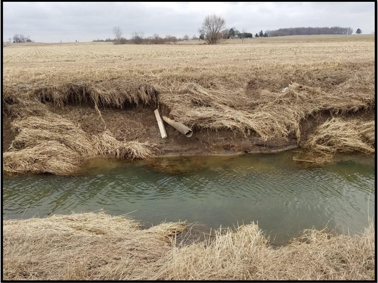
Figure 23: Severe ditch bank erosion along an intermittent stream in Crawford County. Erosion as severe as this can be a safety hazard and is a source of sedimentation in downstream reaches, and a possible nutrient runoff site from adjacent crop fields.
