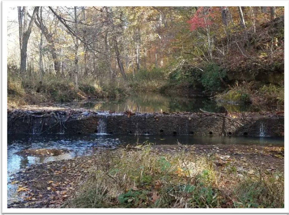
Figure 9. Low-head dam located in Critical Area 1: Big Sandy Run. Photo Credit: Brooke Sanderson (Ohio University)
