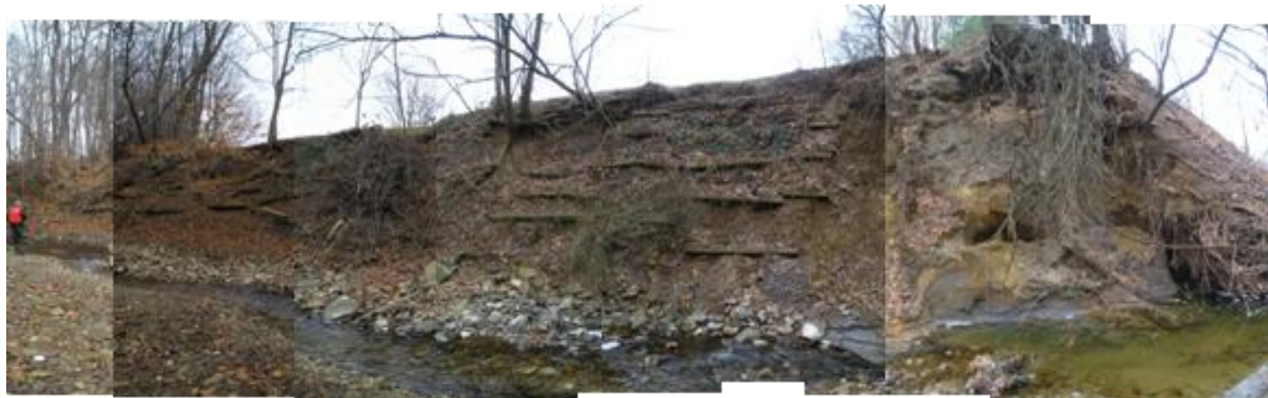
Figure 12: Stream Bank Erosion in Dysar Run
