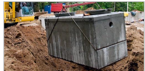
Industrial wastewater holding tanks or pretreatment systems require a permit-to-install from Ohio EPA.
