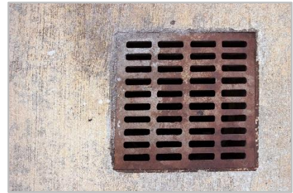
Label floor drains and consider having them capped or plugged if not in use.
