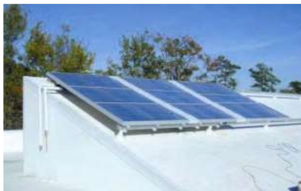
Solar collectors mounted on north-facing roof monitors
