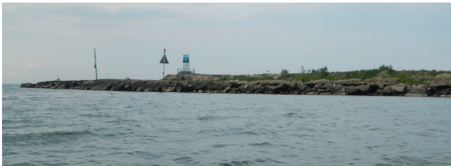
A nearly continuous armor stone revetment protects almost 4 miles of shore lakeward of the Norfolk Southern Railway at the east end of the City of Vermilion and the west end of the City of Lorain (top). The revetment is split near the center by the jetties at the mouth of Beaver Creek (bottom).
