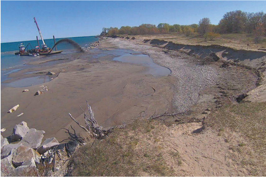
Clean sand dredged from Kenosha Harbor in Wisconsin is pumped to a beach placement site. Chin Wu
