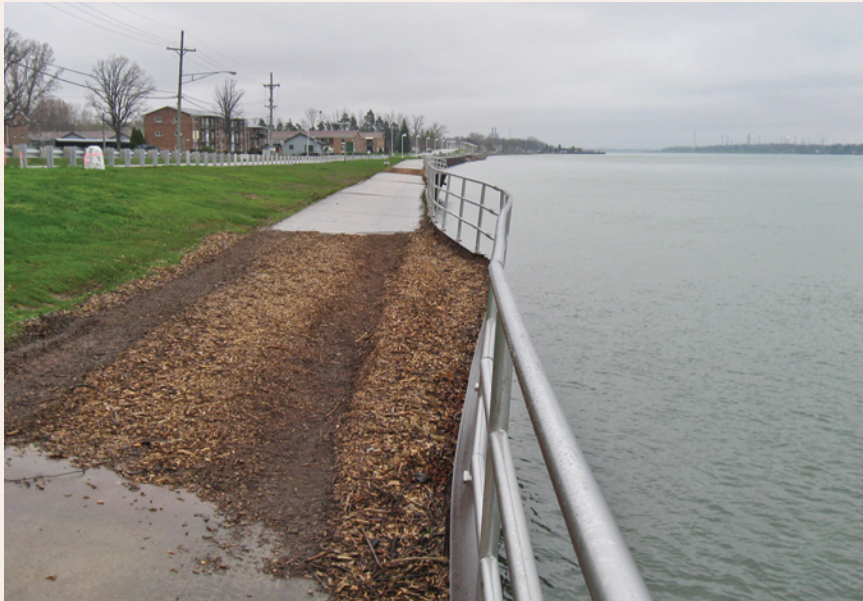
Before The area was protected with a steel sheet pile seawall that had become unstable and provided limited environmental benefits. Barry Kreiner
