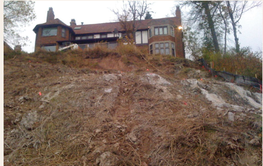
Before Before stabilization, the bluff was failing very close the residence, indicated by the steep unvegetated slope close to the home. Marek Landscaping
