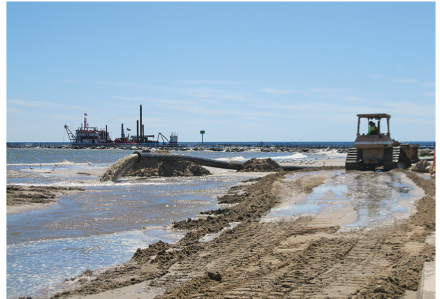
Clean, coarse-grained sediment dredged from the Two Rivers Harbor in Wisconsin is pumped to the placement site and spread across the beach with heavy machinery. Jim Killian
