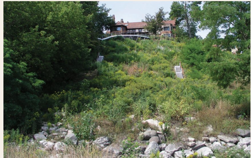
After Stabilization of the upper slope incorporated native vegetation, improving the aesthetic and recreational value of the property. Marek Landscaping
