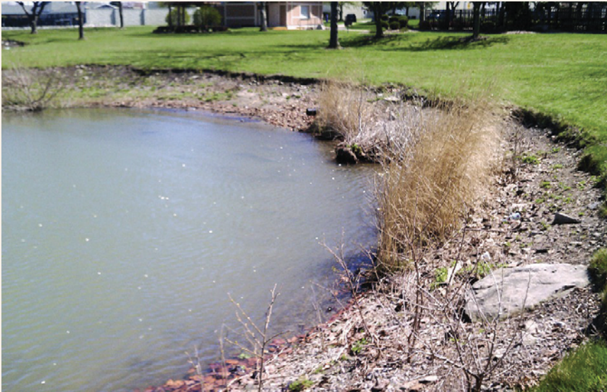
Before A turfgrass shoreline was eroding and visually unappealing. Erie Soil and Water Conservation District
