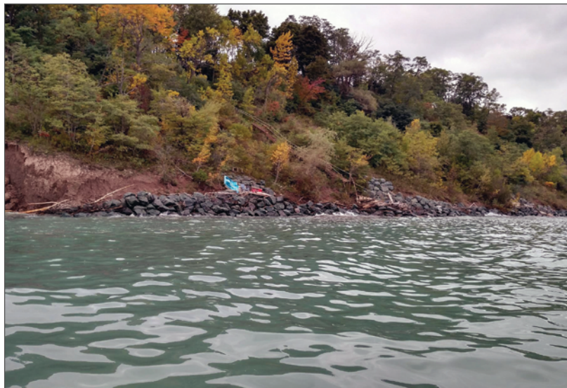
LEFT Flanking around the unprotected end of the revetment has led to accelerated erosion. Chin Wu RIGHT Overtopping of this revetment has led to erosion on the back side of the armor stone. Adam Bechle
