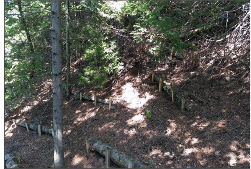
Brush and logs staked in to the bluff to slow the flow of surface water runoff. Adam Bechle
