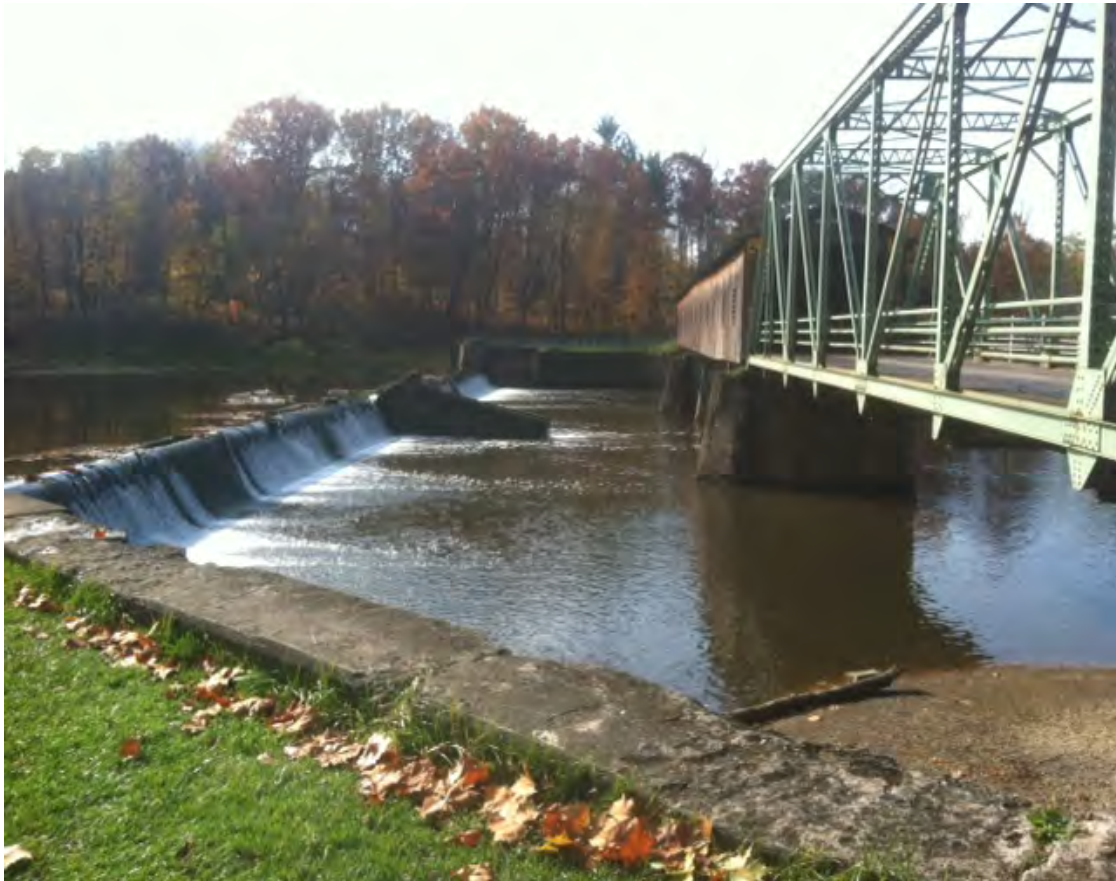
Harpersfield Dam on the Grand River The dam has served as a barrier to the upstream migration of Sea Lampreys. Photo: ODNR
