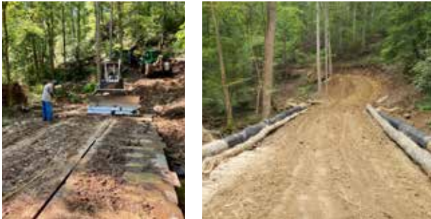
Figure 25. A steel skidder bridge under construction. After placing and securing the steel panels, filter fabric was placed over the panels to keep sediment from falling into the stream. Wood mats were then placed over the fabric as a wear surface.
