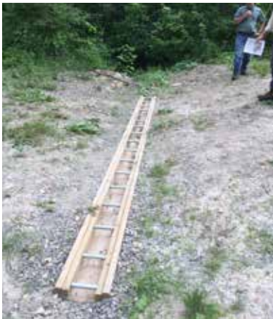
Figure 32. An open-top box culvert used as an alternative to a water bar on a closed trail. These structures are very effective but require routine maintenance to remove leaves and other obstructions.
