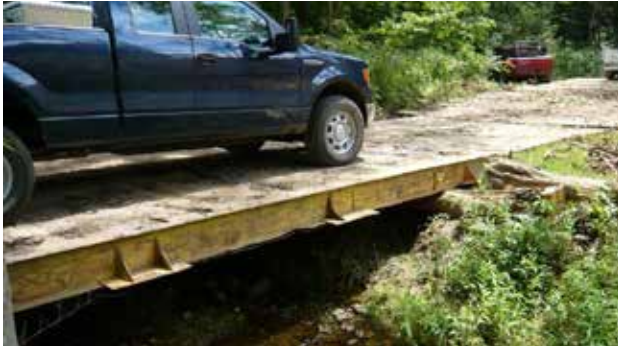
Figure 24. A properly installed haul road bridge. Note the use of wood mud mats to armor the approach.
