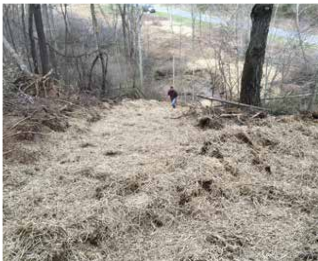
Figure 36. A steep skid trail that has been seeded and mulched. Note the water bar in the foreground.
