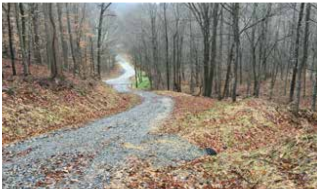
Figure 15. A well-designed haul road. Note the use of culverts for water diversion. Culverts should cross the road at approximately 30-degree angle downgrade to ensure adequate fall (see Figure 18 for installation details).
