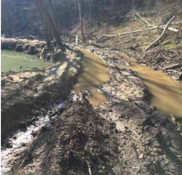
Figure 13. An improperly placed skid trail that has damaged the SMZ and created a water quality violation. Note the absence of any mitigating BMPs.
