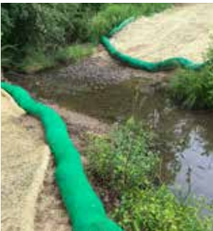
Figure 9. A temporary composting filter sock sediment barrier that is filled with wood chips. Filter socks generally require less labor to install than bales or silt fence since they can be placed directly on the ground without a trench. This also makes them a good choice when the ground is frozen or rocky.
