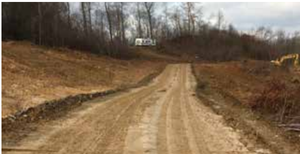
Figure 19. Portable wood mud mats being used to create a temporary road surface through a wet area.
