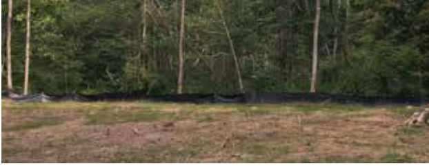
Figure 7. A properly installed silt fence is a cost-effective way to control sedimentation from large, disturbed areas, such as log landings.
