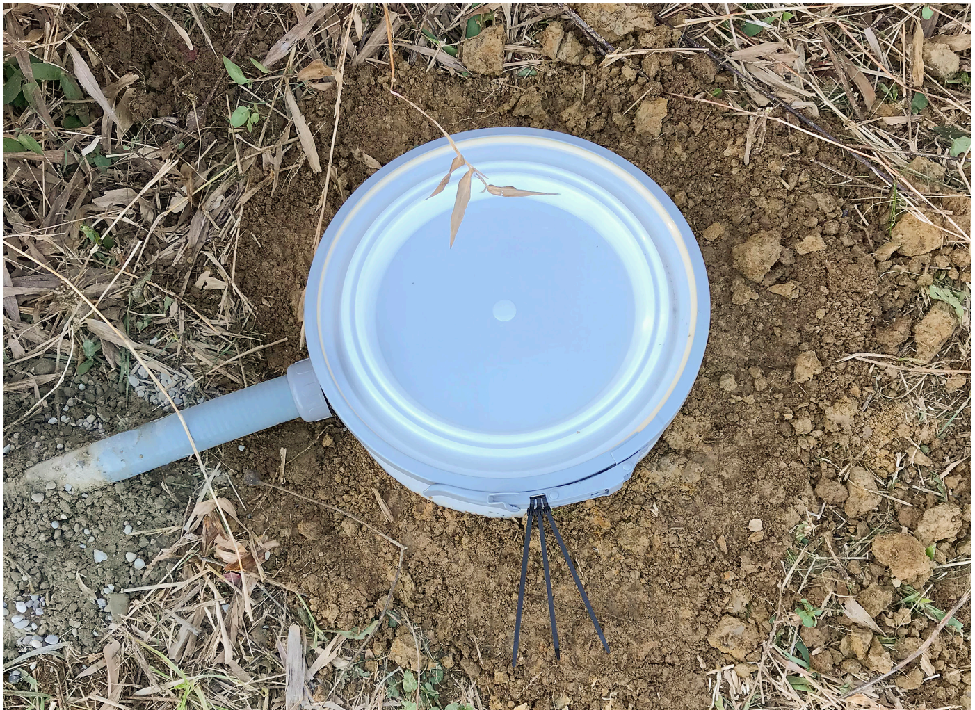
FIGURE A-1. A newly redesigned OhioSeis surface vault, installed in 2020.
