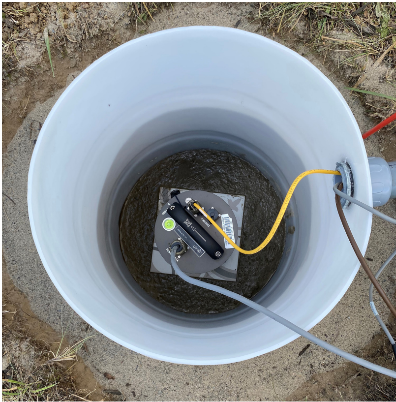
FIGURE A-3. New seismometer vault at Sycamore State Park.
