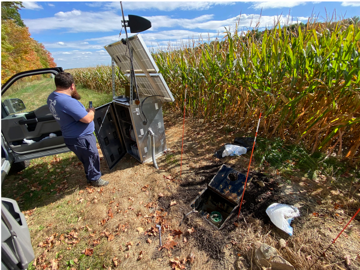
FIGURE A-5. Photo showing Instrument installation and checks at M53A in Trumbull County.
