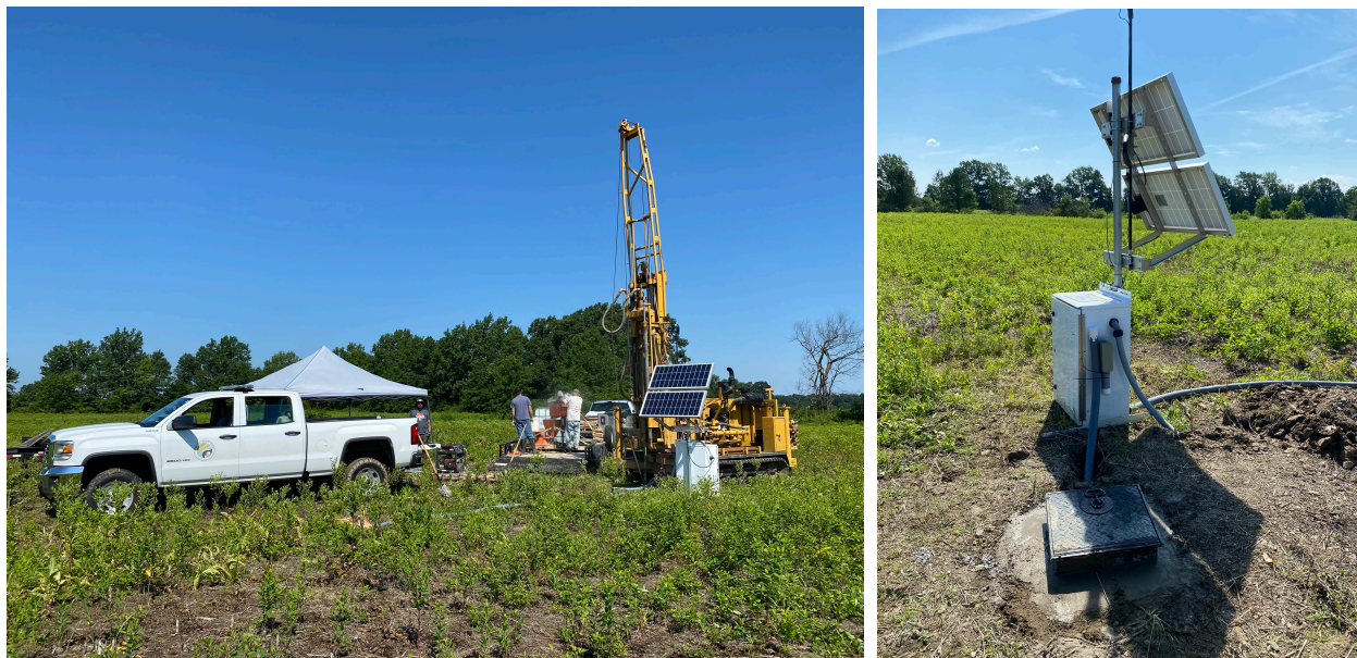
FIGURE A-6. Photos taken at OhioSeis station KDOH at Killdeer Plains Wildlife Area in Wyandot County, Ohio. Left: Drilling borehole for the station. Right: Finished station.
