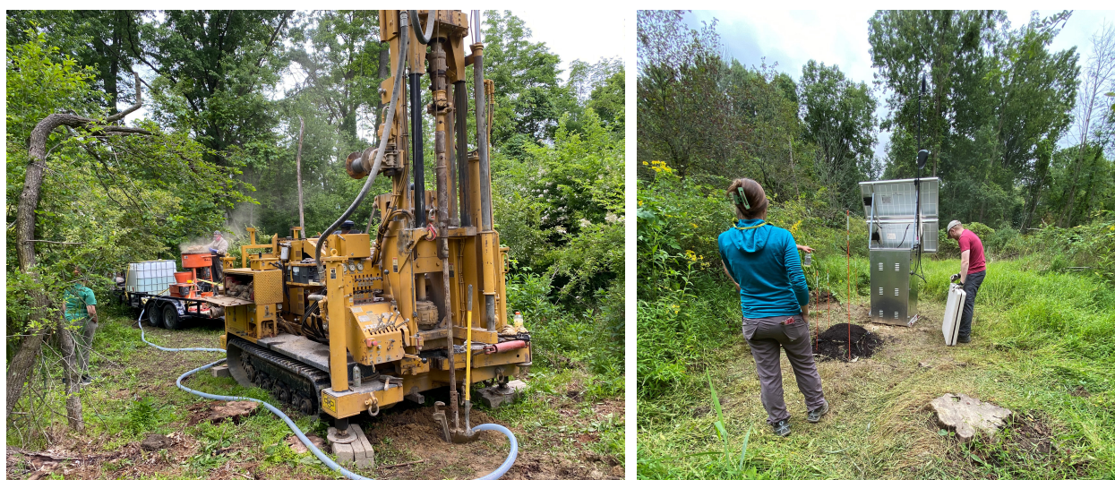
FIGURE A-2. Photos taken at OhioSeis station CHOH at Chagrin River Park in Lake County, Ohio. Left: Drilling at the site prior to installation. Right: Installation of seismic station equipment.
