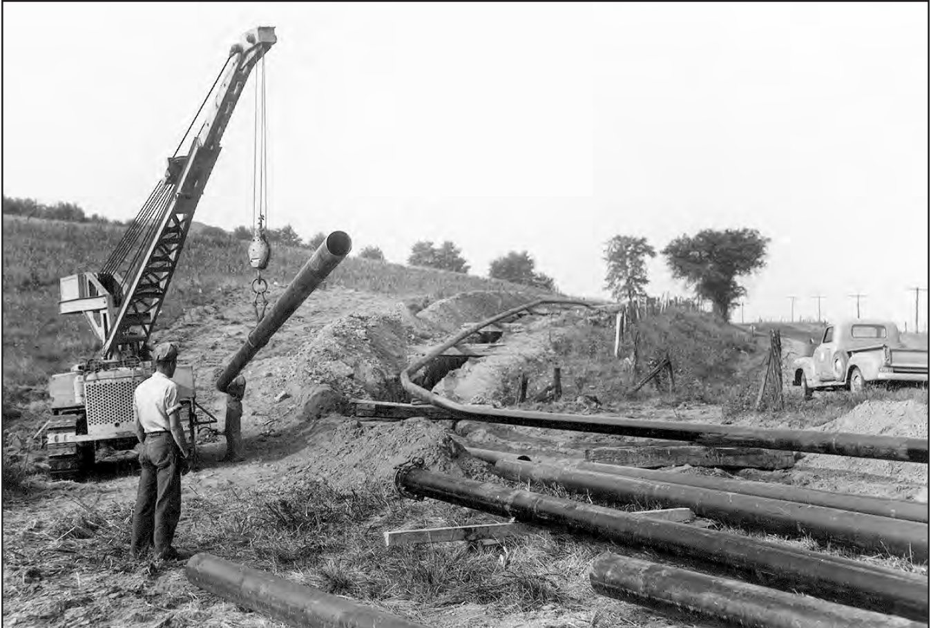
FIGURE 202.—Coal-slurry pipeline under construction in 1956. The 10-inch, 108-mile-long pipeline linked the Hanna Coal Company Georgetown preparation plant (see fig. 203) near Cadiz, Harrison County, with the Cleveland Electric Illuminating Company Eastlake Generating Station in Eastlake, Lake County. This pipeline supplied about 6 million tons of coal to the Eastlake Generating Station from 1957 to 1963. Location unknown. Photo courtesy of Dale Davis.
