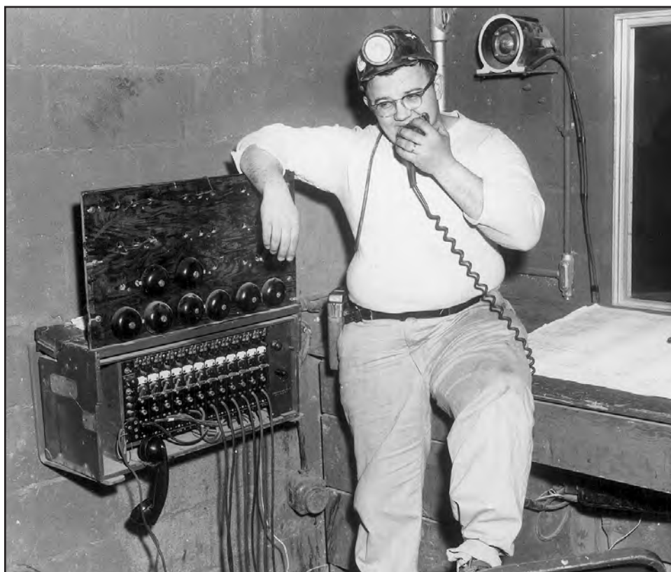
FIGURE 154.—Veteran motorman Joe Graham (top) using a trolley phone, which was standard equipment in the Hanna Coal Company Willow Grove No. 10 mine (Bt-163). On the other end of the line is an unidentified dispatcher (bottom), who, from the radio control room of the Willow Grove No. 10 mine, is advising Graham of current man-trip movements. Trolley phones, similar to walkie-talkies, allow miners several miles apart to communicate with one another and thereby increase safety and operational efficiency. Photo courtesy of Dale Davis, from Hanna Coal News (March 1948, p. 10). (For other photos of this mine see figs. 35, 79, 82, 93, 110, 117, 119, 120, 123, 140-142, 153, 193.)
