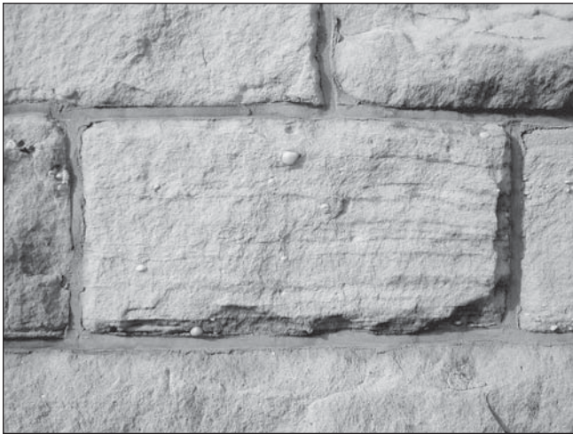
FIGURE 7-6.—Close up of Sharon building stone at St. Vincent Church, downtown Akron. Photo by A. Foos.
