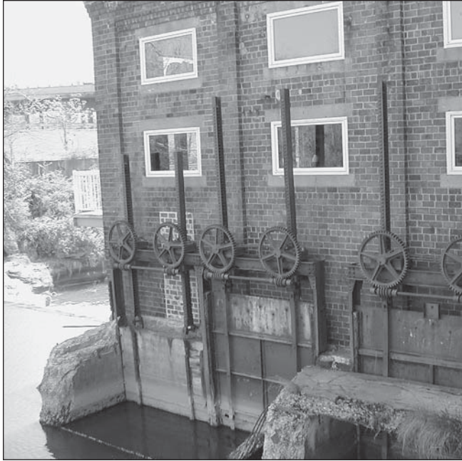
FIGURE 7-3.— The gate mechanism at the inlet to machinery of the old powerhouse, built after the 1913 flood. Le Fever's River Grill in downtown Cuyahoga Falls (2291 Riverfront Pky.). Photo by A. Foos.
