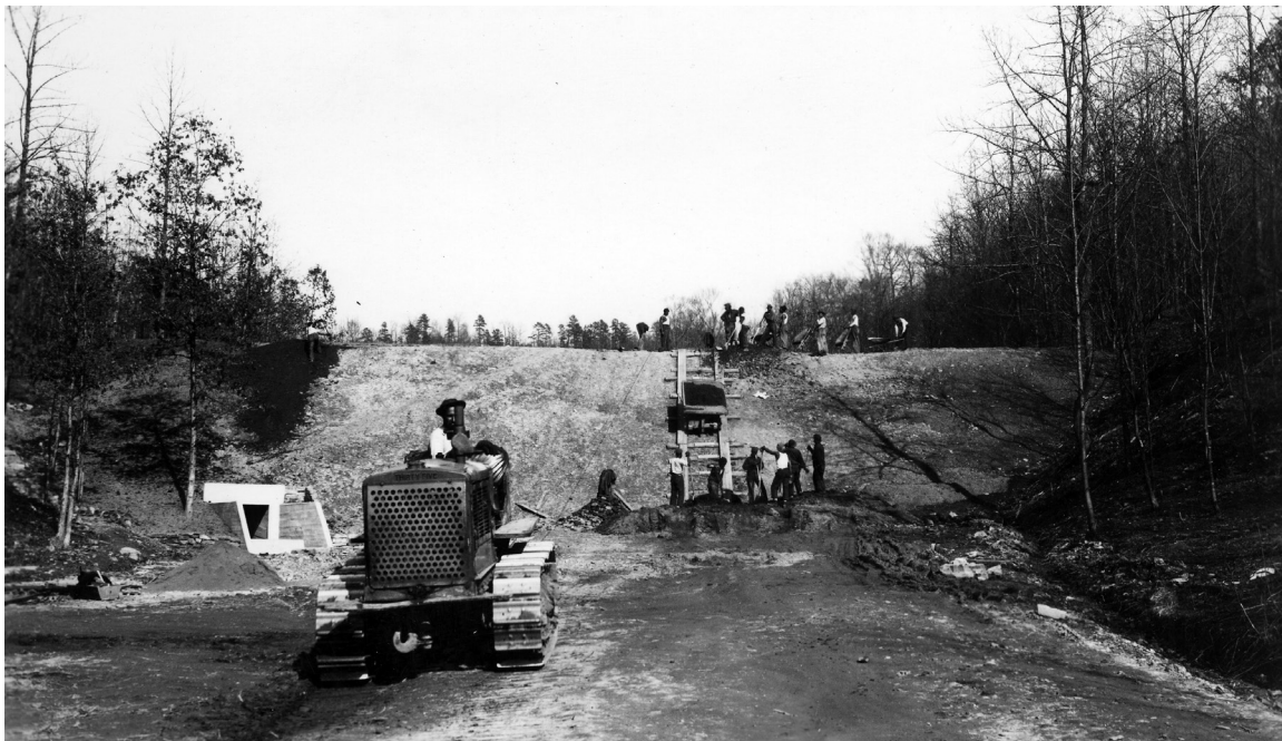
FIGURE 3.—Civilian Conservation Corps crew constructing Churn Creek Lake dam, circa 1930s, Shawnee State Forest, Ohio. Photo from the Ohio Agricultural Experiment Station, Department of Forestry collection at The Ohio State University.
