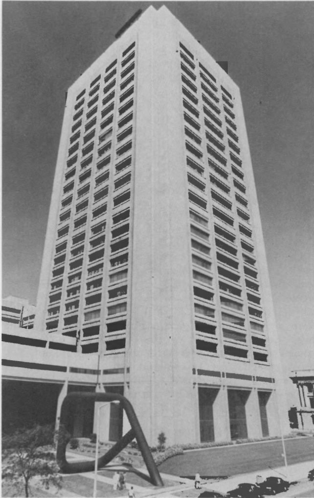
FIGURE 19.—Justice Center. Cracks have developed in the Spanish Pink granite used to face the building and for sidewalks around the building. Photo circa 1988.
