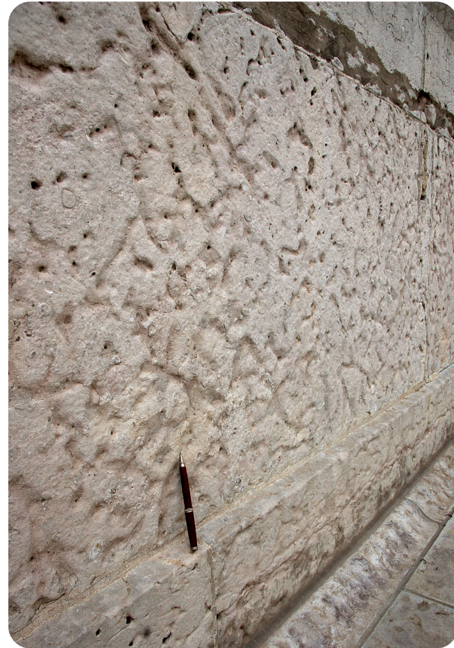
Feeding burrows produced by an unknown type of animal, preserved in an exterior wall of the Statehouse. In places (such as at top right of this photo), Statehouse caretakers have filled exposed burrows with grout to reinforce the facing.
