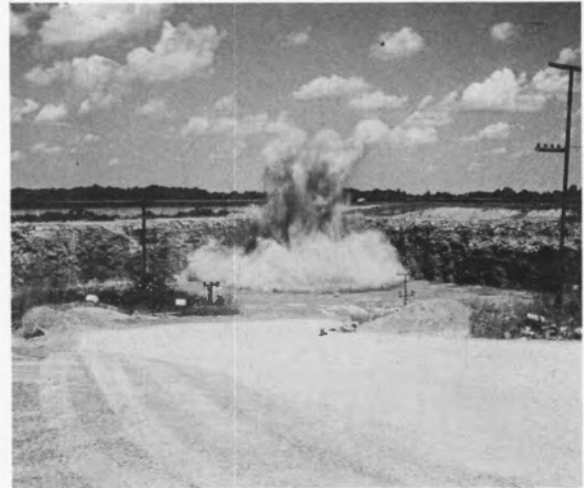
Blasting at limestone quarry at Custar, Wood County, circa 1982 (photo by Robert W. Hites, Jr.)
