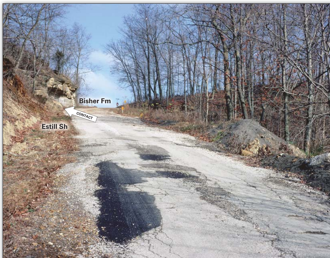
Landslide damage occurring to Poplar Ridge Road in Adams County below the contact of the Estill Shale and the Bisher Formation. Estill Shale clay-rich colluvium is exposed in road cut on left and a cliff of the Bisher Formation occurs in the road cut at the top of the hill.
