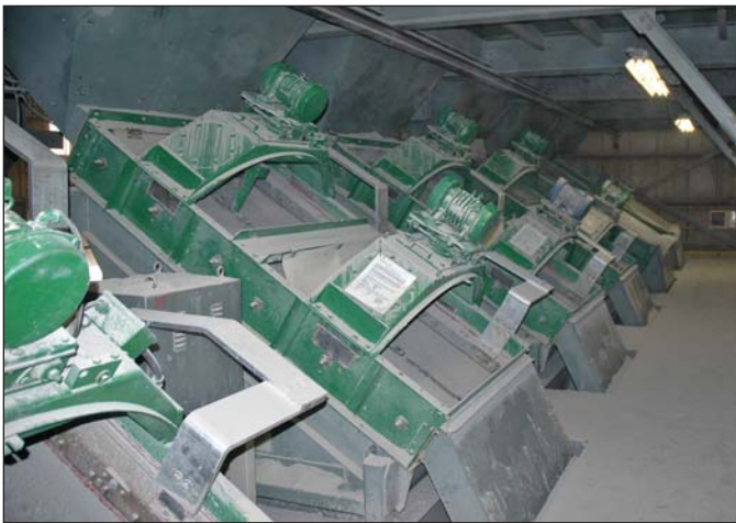
FIGURE 8. Inclined screens used to ensure proper size of clay and shale at the Ironrock/Metropolitan Brick ceramic tile plant located south of Canton, Ohio.
