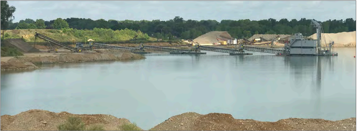
(ABOVE) A clamshell dredge excavates sand and gravel on permit IM-2140 operated by Stoneco, Inc. in Stark County.
