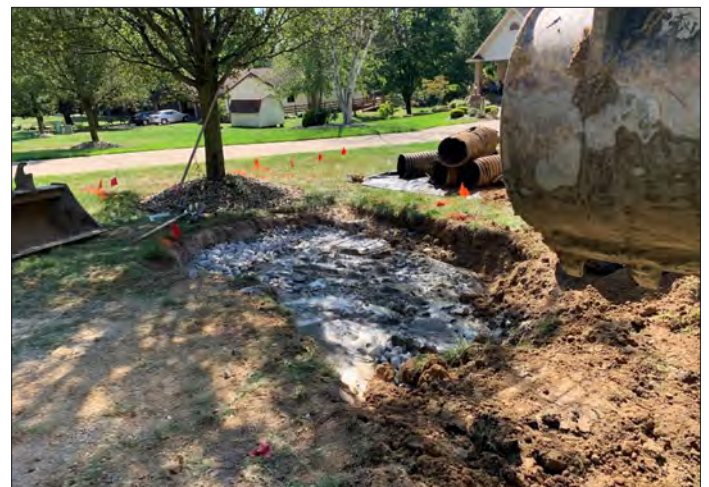
(ABOVE) Images of the Ripplinger Subsidence Emergency site in Wayne County, Chippewa Township show before and during reclamation to stabilize a dangerous subsidence caused by the collapse of an undocumented mine. Information from past projects showed the Sharon #1 coal seam was mined in this area from 1896 through 1912. (TOP) Subsidence adjacent to Hollow Ridge Road. (MIDDLE) Excavated subsidence. (BOTTOM) Grouted rock plug installation.
