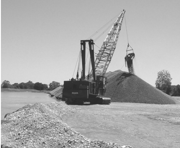
A dragline is used to excavate sand and gravel deposits below the water table.
