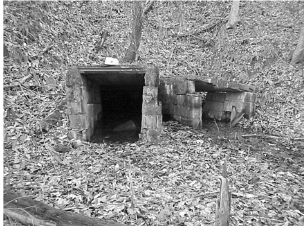
A potentially dangerous deep mine portal opening remains as evidence of past mining activity.
