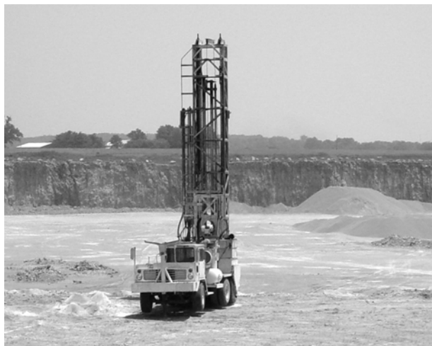
Drilling activities in preparation for blasting. Holes will be loaded with explosive charges.
