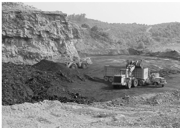
Removing and loading coal at a surface mine. Such sites are inspected on a regular basis for compliance.
