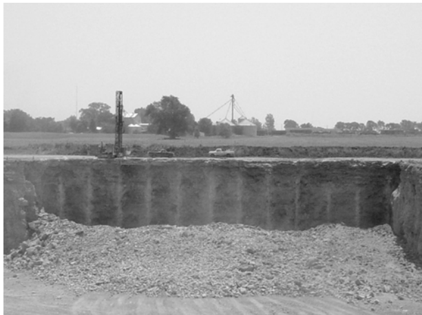
After a blast, the active face of this mining operation shows evidence of the drilling holes above the most recent pile of shot rock.
