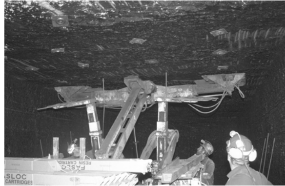
Underground miners install roof bolts in the ceiling of an active underground mine.
