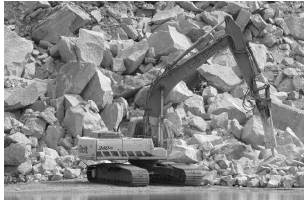
A backhoe-mounted jackhammer breaks massive pieces of limestone into smaller stone for processing.
