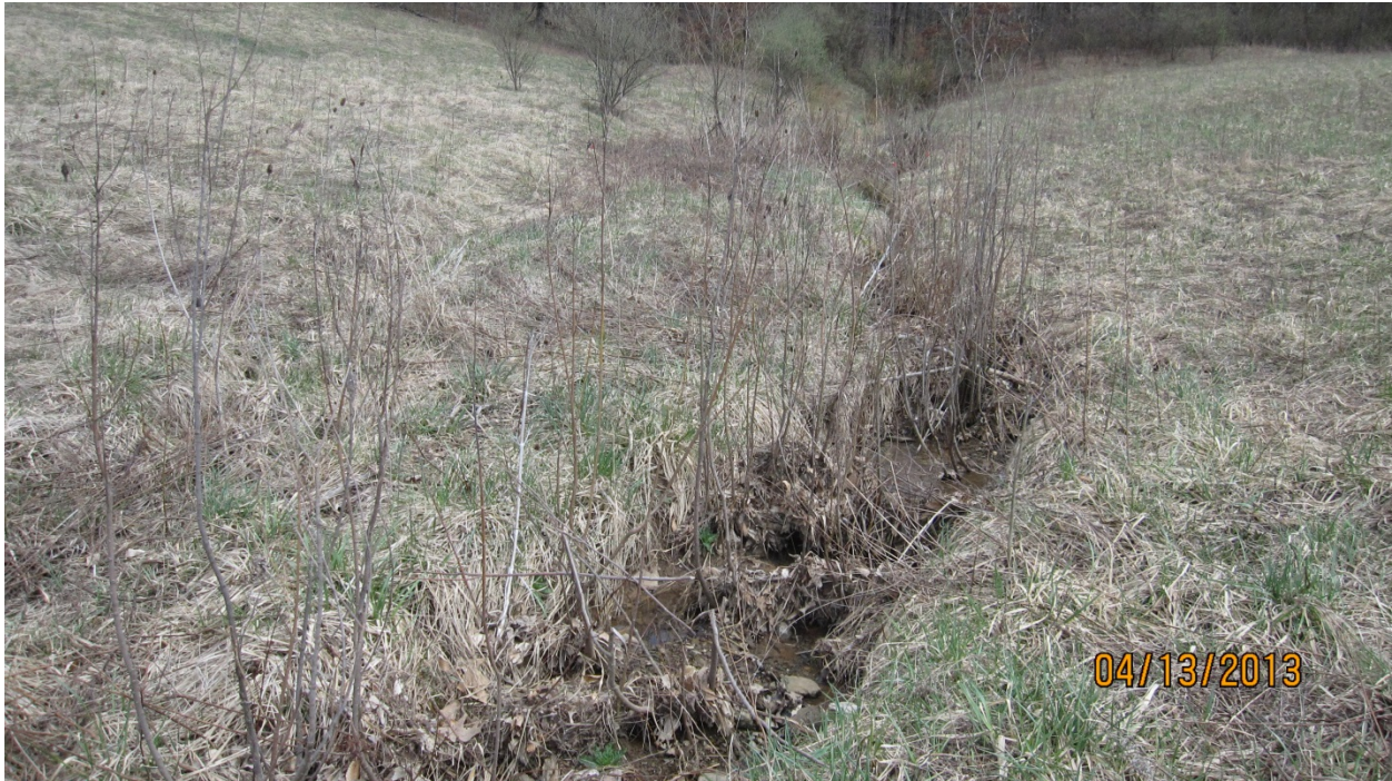
D-0807– view of substrate near the upper end of reconstructed stream segment
