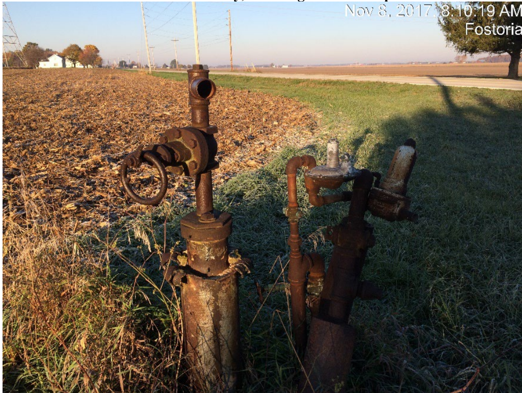
Marvin Kelbley #1 wellhead
