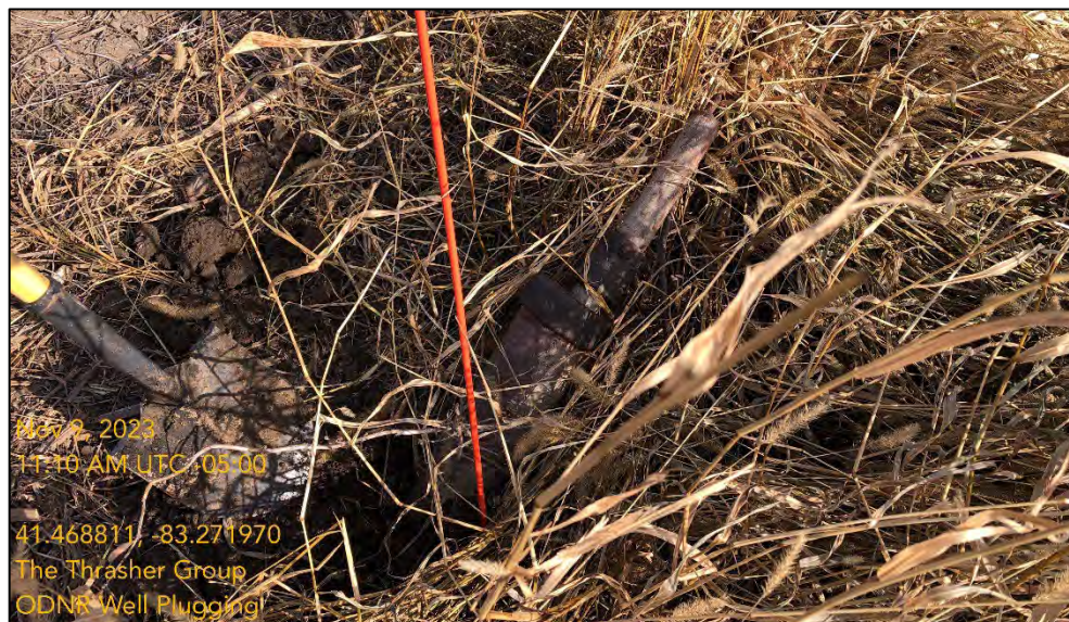
Photograph # 2: Knipp 9 (Water Well)
