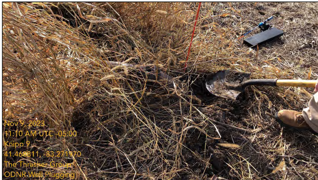
Photograph # 1: Knipp 9 (Water Well)
