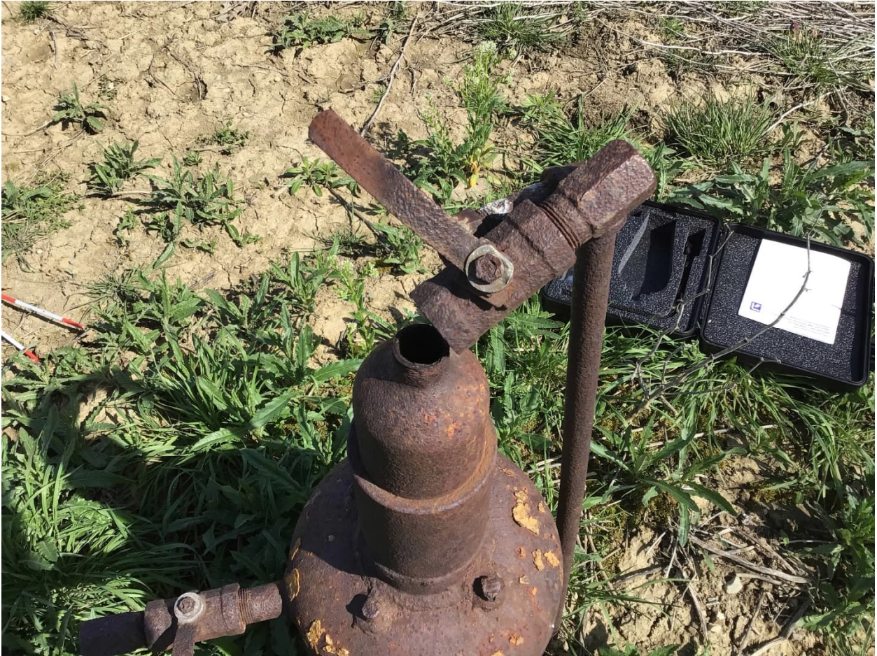
View of well casing and valve, note valve is broken and well is venting to the atmosphere.
