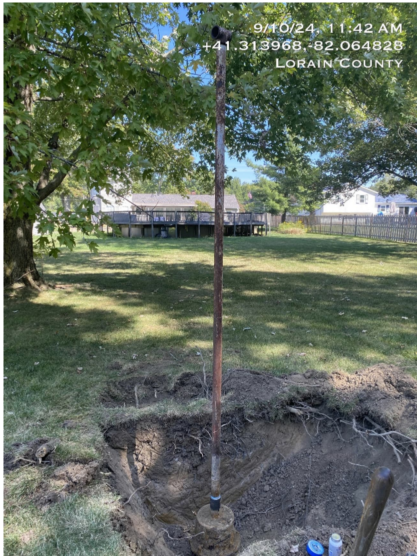
View looking north of well head and vent pipe. Well was further east than initially thought.
