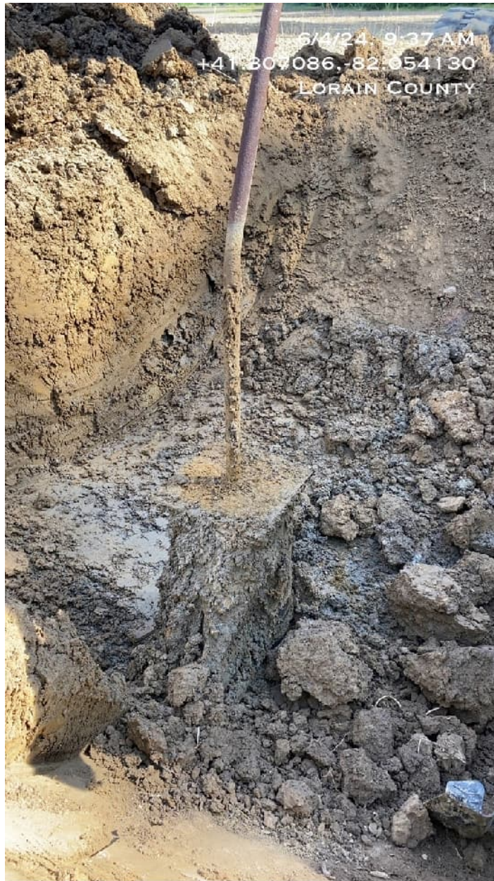
2024 photo of the Carpenter-Yost #1 showing the 1-inch diameter tubing welded to the diamond plate covering the 11-inch diameter casing.
