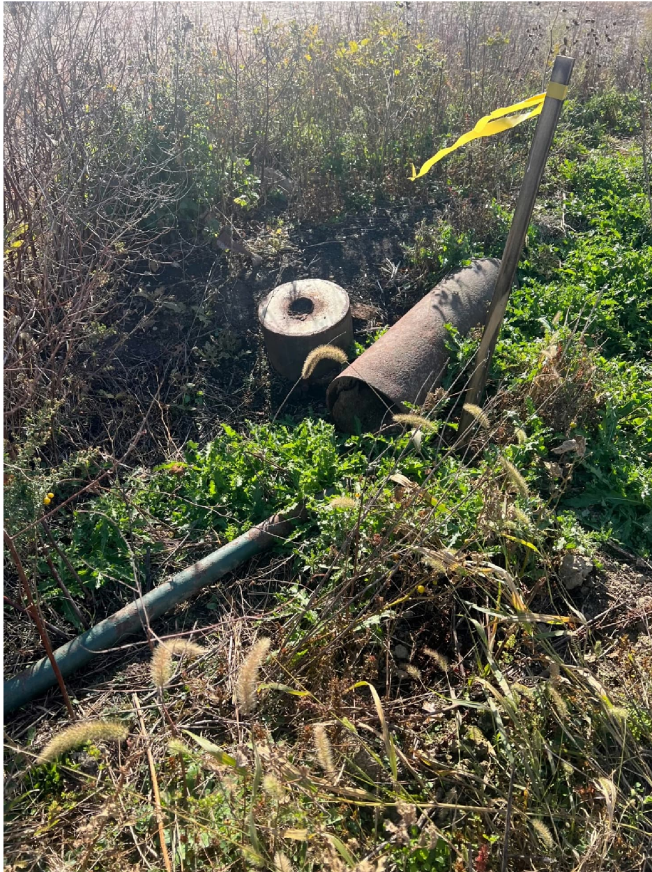
View of well and vent disconnected from the well. Well is currently venting to the atmosphere.
