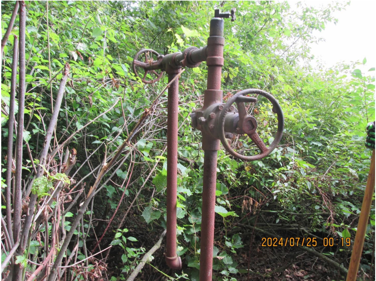
View of valve assembly and flowline.
