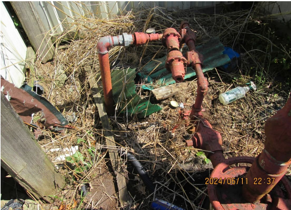
Photos of the Kantosky C&B #1 showing the 2-inch diameter production tubing exiting the top of the well head, the domestic service line connected to one of the ports in the well head (top photo) and the 2-inch diameter flow line connected to second port of the well head (bottom photo), with their associated valves, regulators, and gauges.
