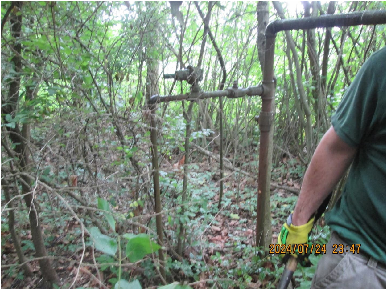
Spitzer Ford Agency #1 domestic line looking west.
