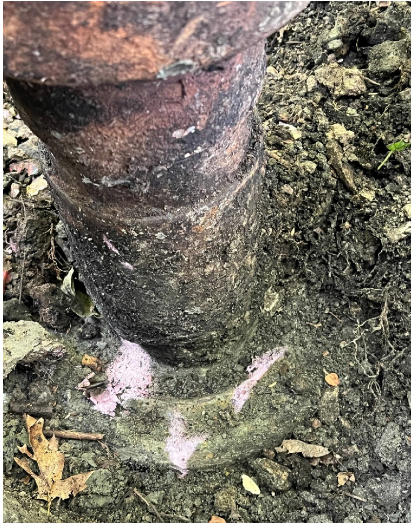
July 2024 photo of the Spitzer-Jackson #1 (API# 34-093-2-0946-00-00) showing the exposed surface casing head, which was found approximately 8 inches below grade.
