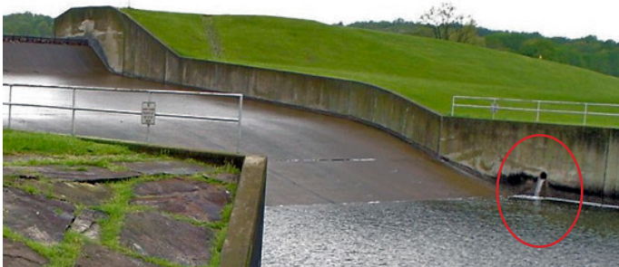
A properly designed spillway includes a drainage system for collecting seepage under the spillway. The picture shows flow discharging from the spillway's drainage system.
