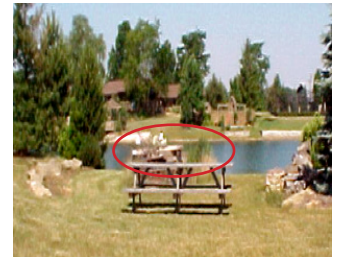
Notice the landscaping directly behind the table. Obstructions in the spillway reduce the capacity to convey water. They also can collect debris, further diminishing the capacity of the spillway.
