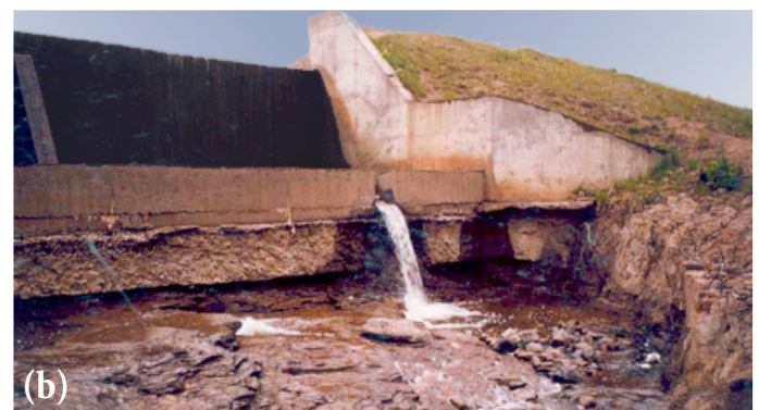
(a) A spillway outlet area as originally constructed. (b) Severe erosion has undermined the spillway outlet and threatens the overall structural safety of the spillway.
