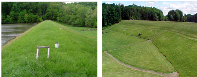
An excellent grass cover will reduce erosion and is easily maintained.
