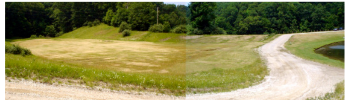
This open-channel emergency spillway is clear of trees, brush and other obstructions. Also note the good grass cover.
