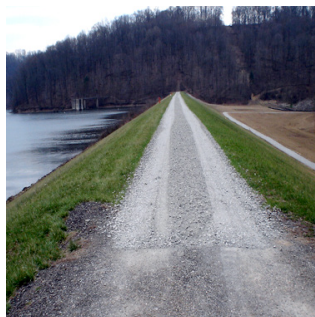
Crest with a good cover that will reduce the effects of vehicular traffic.
