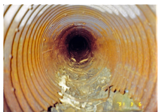
This corrugated metal pipe has corroded completely through the bottom.
