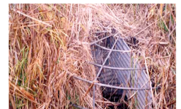
Good trashrack almost completely blocked with vegetation.
