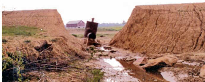
This Dam failed from seepage along the principal spillway.
