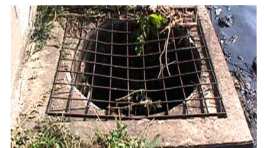
Flat trashracks can quickly become clogged with debris. Also notice the encroaching vegetation.
