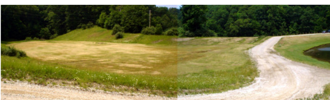
This open-channel emergency spillway is clear of trees, brush and other obstructions. Also note the good grass cover.
