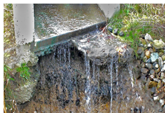
A spillway outlet with inadequate erosion control can lead to undermining of the outlet and failure of the dam.
