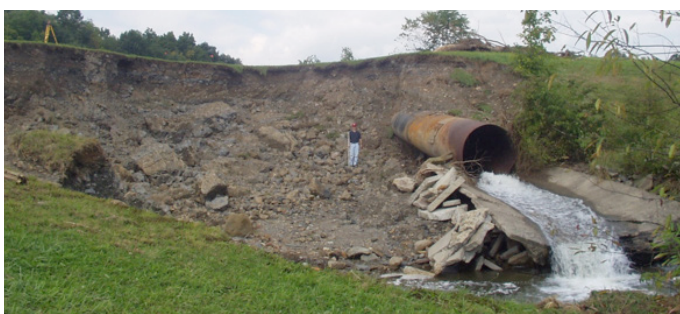
Severe erosion and near failure of the dam (2004) resulted after the principal spillway plugged during a storm. The dam did not have an emergency spillway. The dam was removed one week later.
