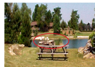
Landscaping, directly behind the table, is obstructing the spillway reducing the capacity to convey water. It also can collect debris, further diminishing spillway capacity.
