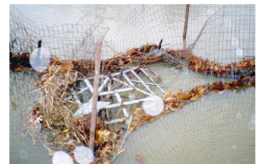
Trashracks with openings that are too small cause leaves to clog the inlet – fencing should not be used.
