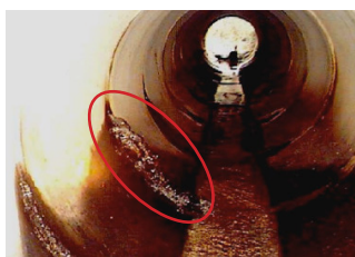
Leaking joints can cause the soil outside the pipe to erode and the spillway to fail.
