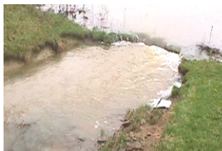
Earthen channels spillways that flow often or continuously will erode. This can eventually cause the dam to fail.
