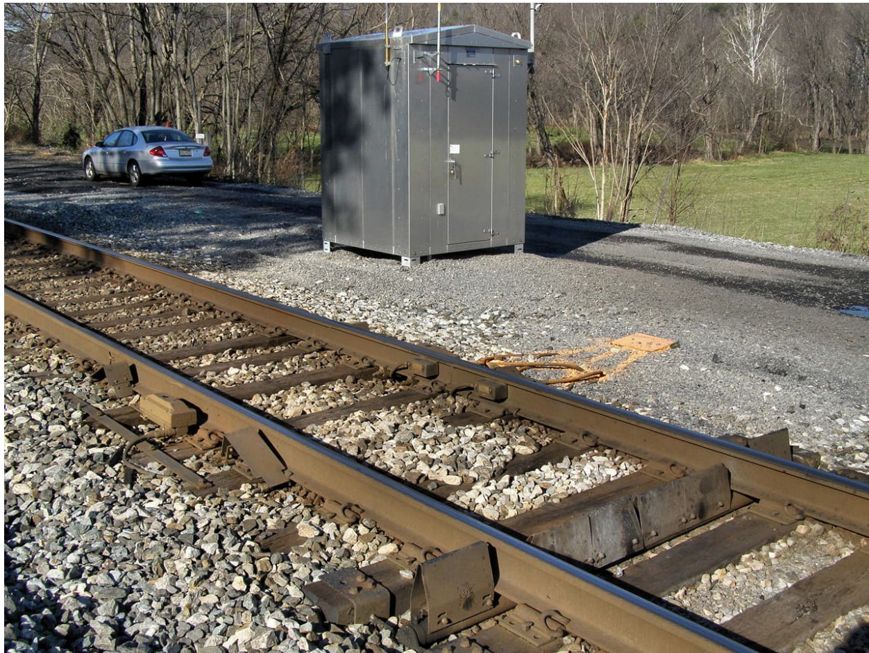
Figure 4-13. Hot Box and Dragging Equipment Detector
