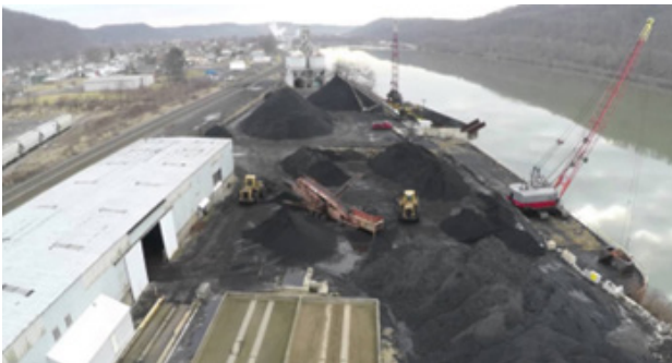
Figure 55: Columbiana County Wellsville Terminal Transloading Equipment Funded Through MAP
