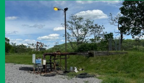
Receiving Pipeline at QLF Facility
