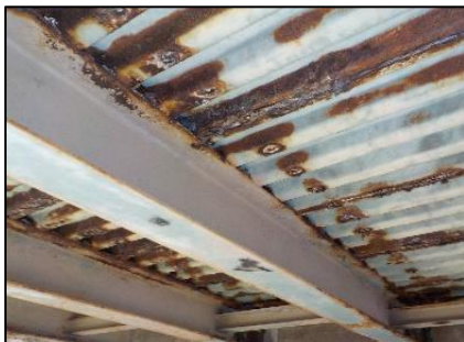
Figure 7-168: Typical areas of section loss near beam interface
