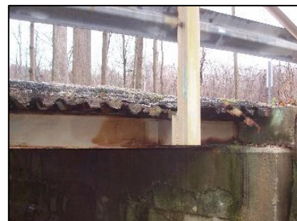
Figure 7-169: Typical edge corrosion
