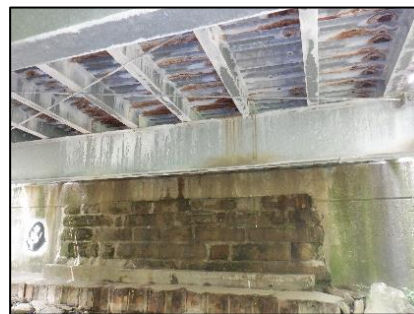
Figure 7-165: Typical widespread corrosion throughout the underside of the deck
