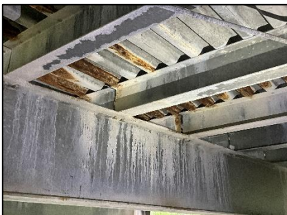
Figure 7-164: Typical underside of deck near drain hole locations
