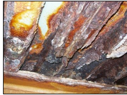
Figure 7-167: Significant section loss to the underside of steel deck pan
