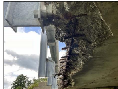
Figure 7-273: Underside of deck along the right edge
