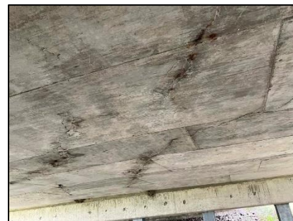
Figure 7-267: Underside of the slab in Span 3
