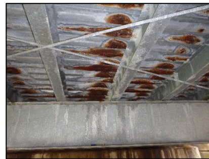
Figure 7-163: Typical underside of deck near drain hole locations
