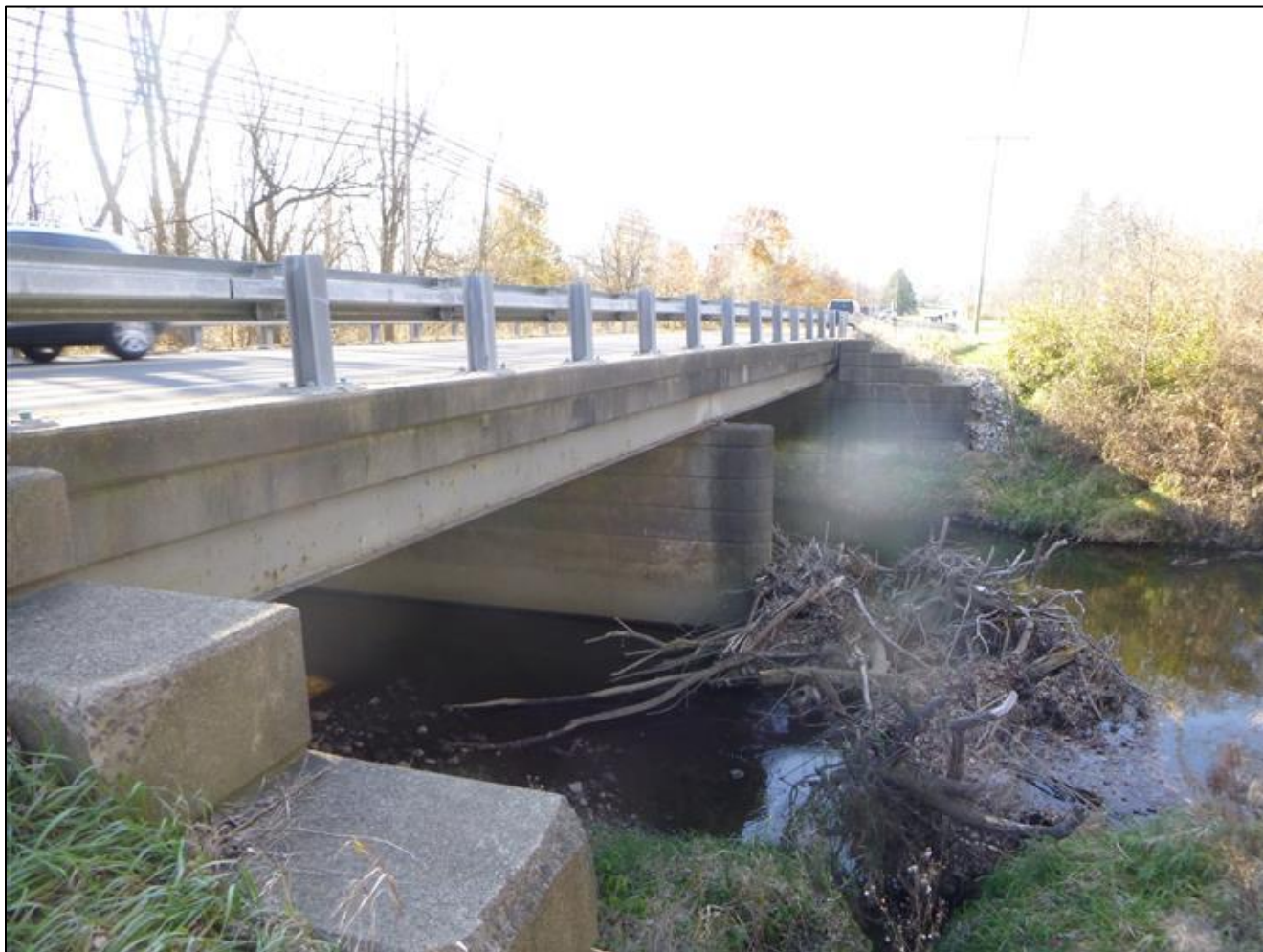
Figure 6 - Heavy Debris will promote scour
