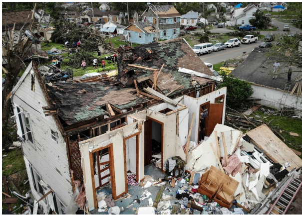
Figure 36: Repair and cleaning efforts begin on a neighborhood damaged by a tornado system that destroyed homes and cut off access to utilities in Dayton, Ohio. (John Minchillo/AP)
